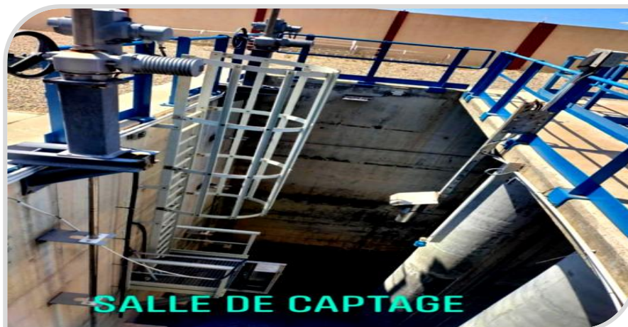
Figure III-2: Salle de captage.
