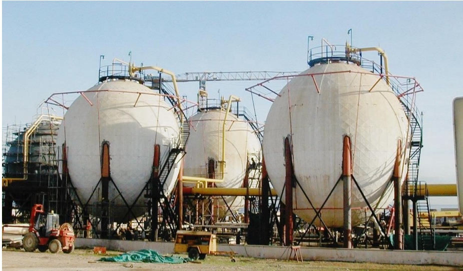
Figure I.5 Sphères de stockage
